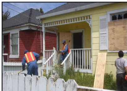
Secure vacant structures.
